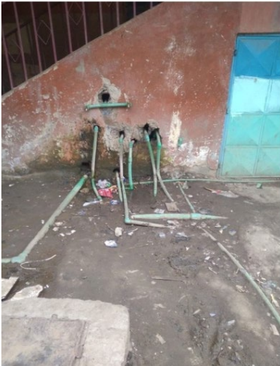
Figure 4. Informal waterpipe connections to increase (democratise) access to water among ghetto residents in Nairobi.
